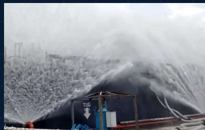
Deluge system test
